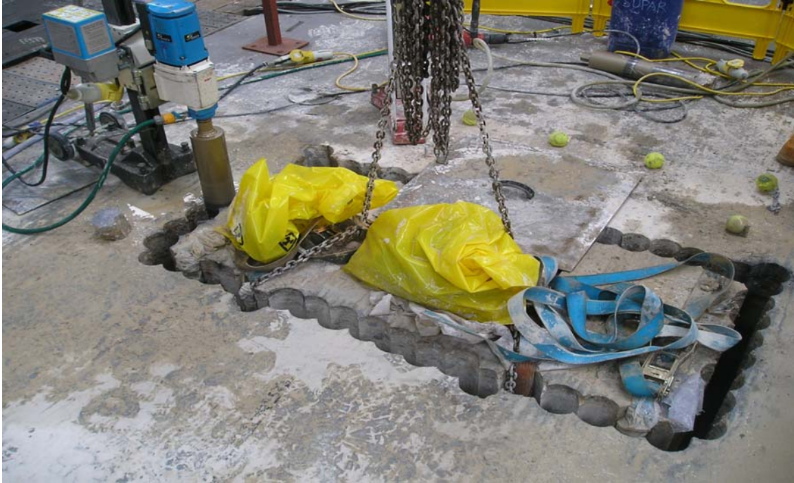
Figure 3: Stitch Drilling an Opening at Tank 1 Roof Position for Sludge Filtration Vessel
