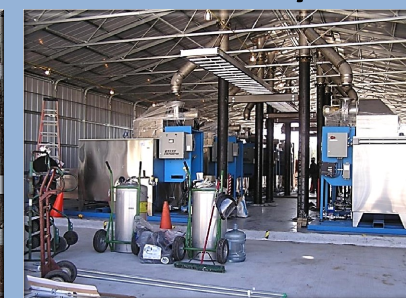
Evaporators in 710-C Evaporator Building
