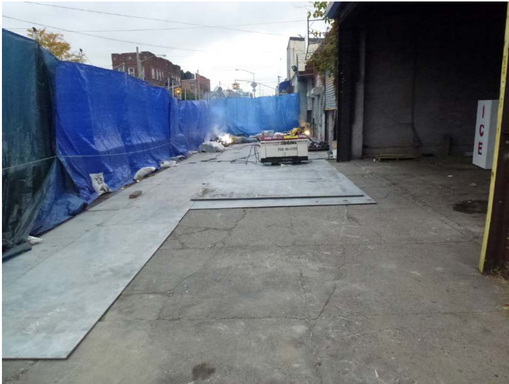
Fig. 6. Installation of steel plates as parts of the radiation shielding on Irving Avenue public sidewalk
