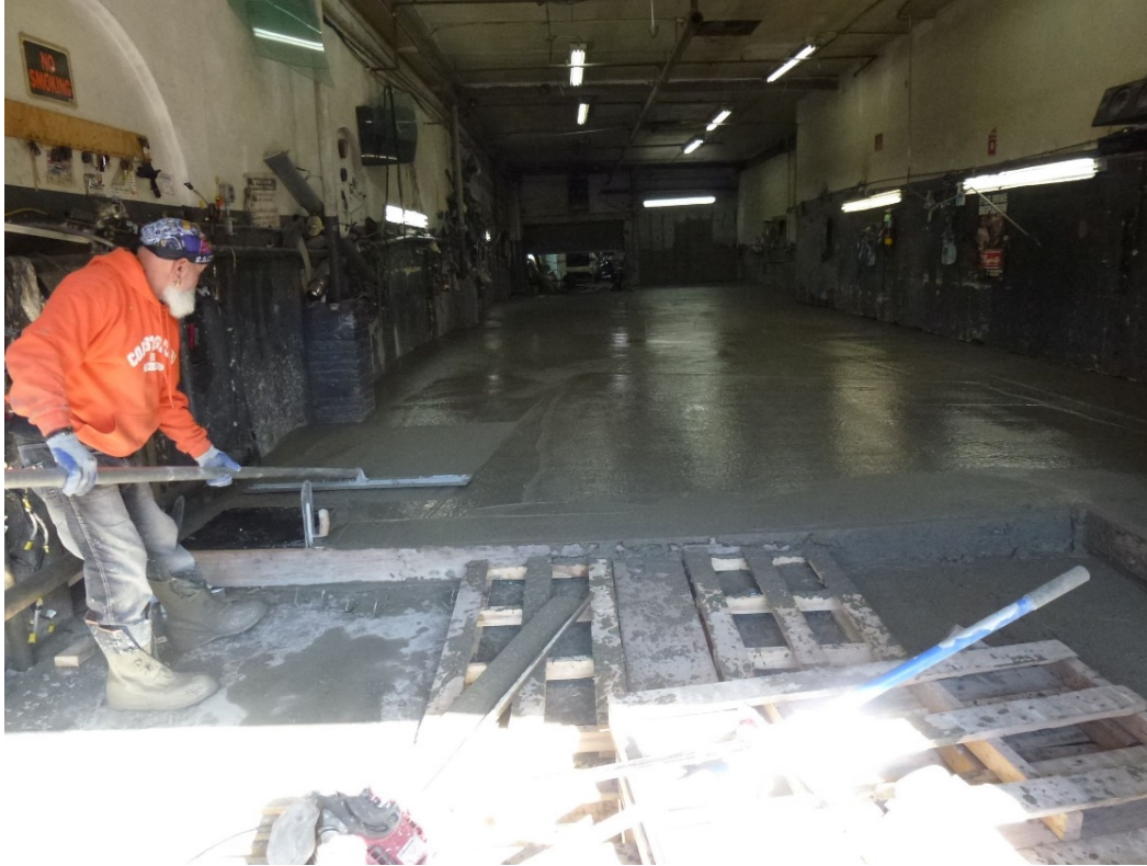
Fig. 7. Application of concrete pad as part of the radiation shielding inside auto repair shop's building
