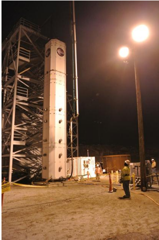
Figure 3. Tall Column Installed at the Cold Test Facility being filled with Simulant
