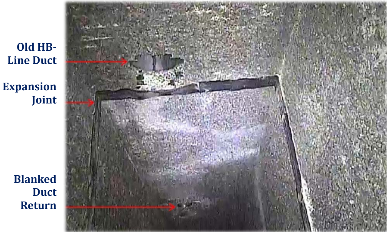
Fig. 18. Duct and Expansion Joint
