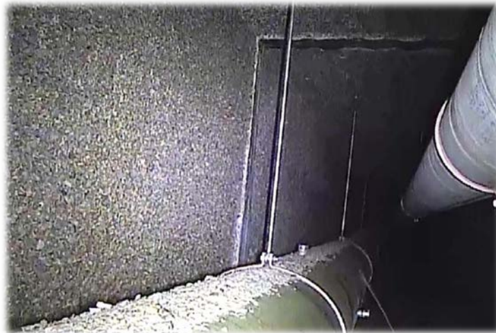
Fig. 19. Other Expansion Joints and Falling Debris on Duct-Work
