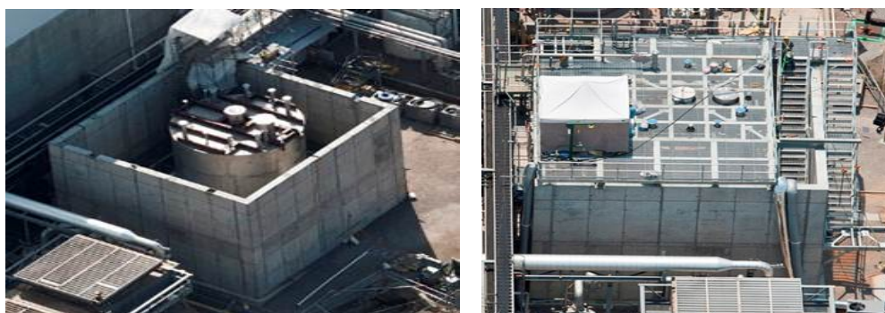
Figure 2. New Waste Concentrate Hold Tank at the Effluent Treatment Facility
