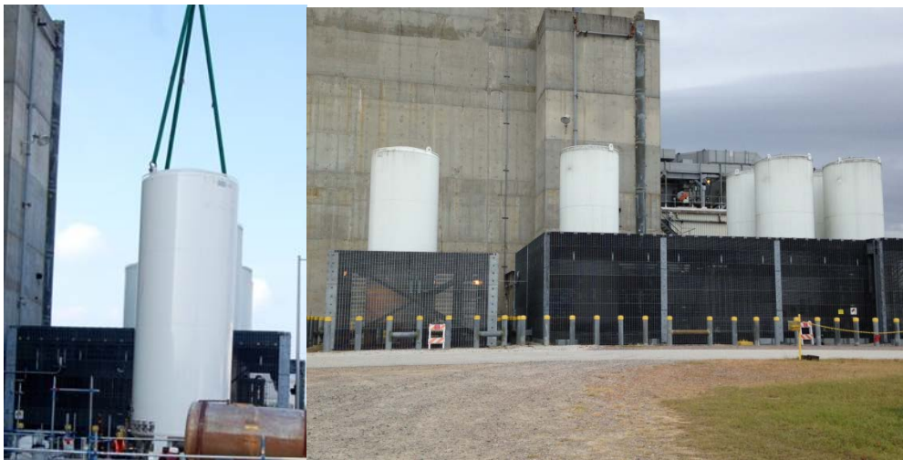
Figure 6. New Nitrogen Storage Tank at DWPF
