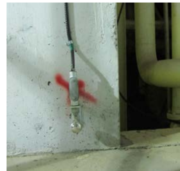
Figure 6: F Reactor Moisture Sensor
