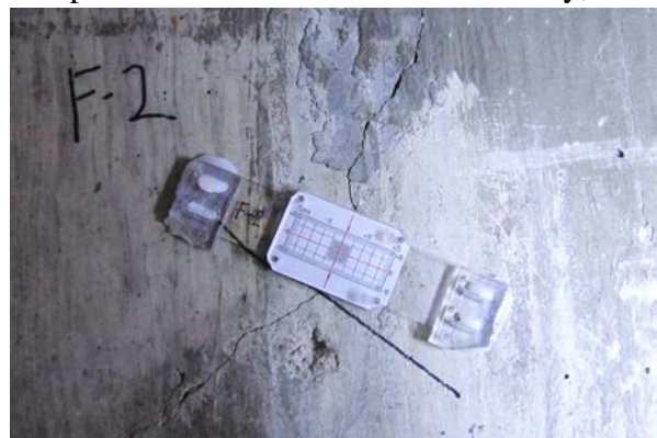
8 Figure 7: Crack Monitoring Gauge Installed at F Reactor
