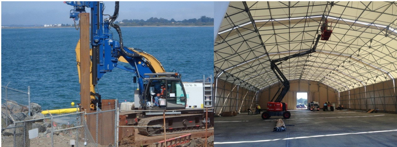
Preparing for Major Civil Works Installation of coffer dam at discharge canal and tents to manage wet canal sediment
