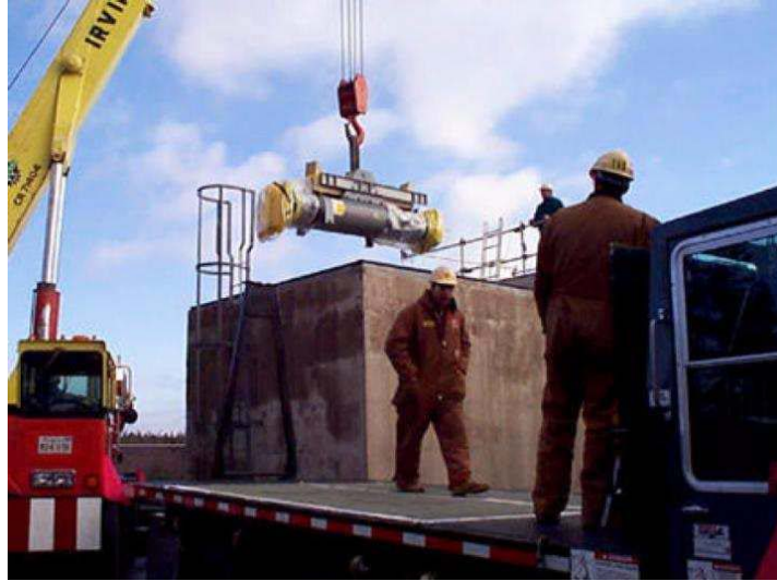
Figure 9 – Filter Flask and Filter Storage Vault
