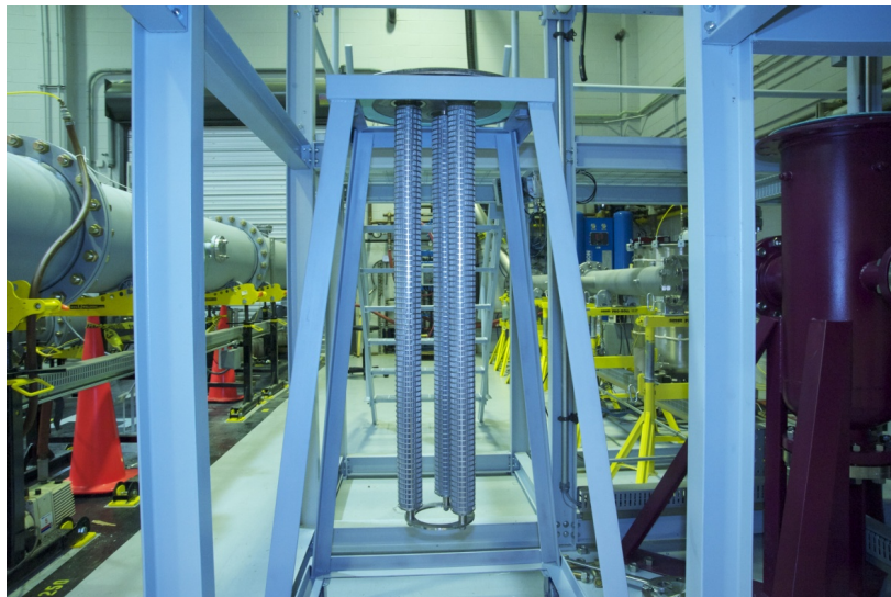
Figure 8. Representative Section FI HEPA Filter Elements
