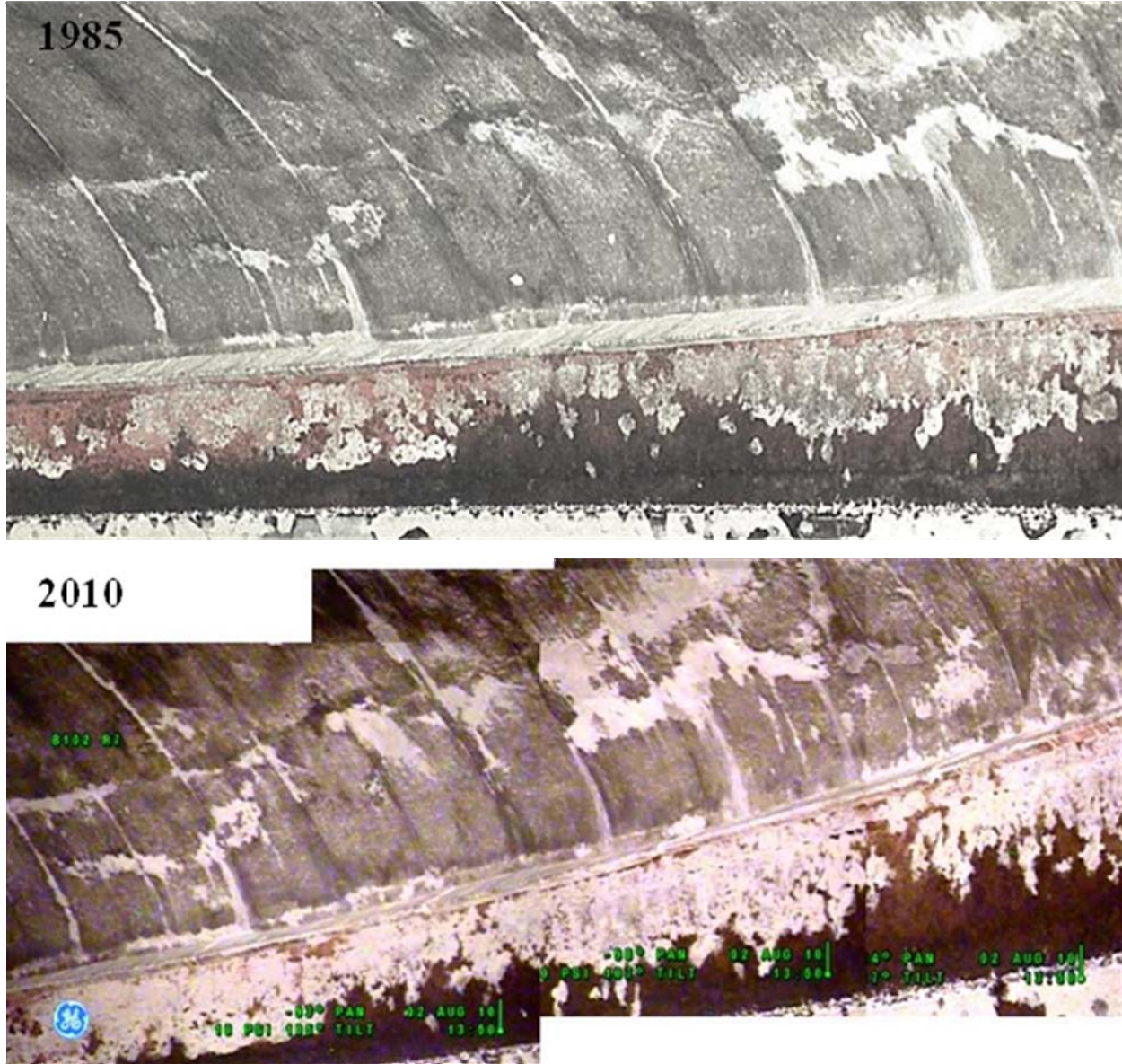
Fig. 3. Comparative Photographs of Tank 241-B-102 Haunch Region
