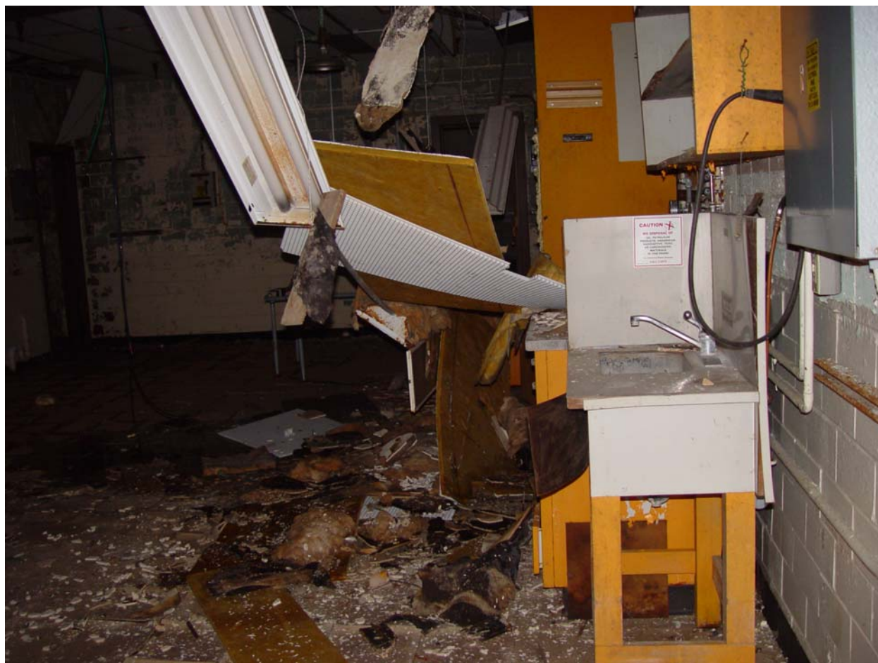
Fig. 4. Sample of interior deterioration in Building 2000.
