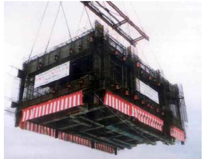
Main Control Room Module - Hitachi
