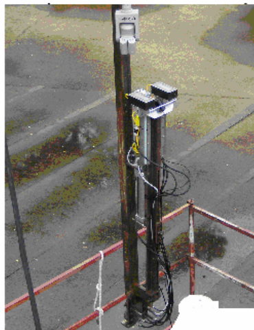
Sampler and mast assembly
