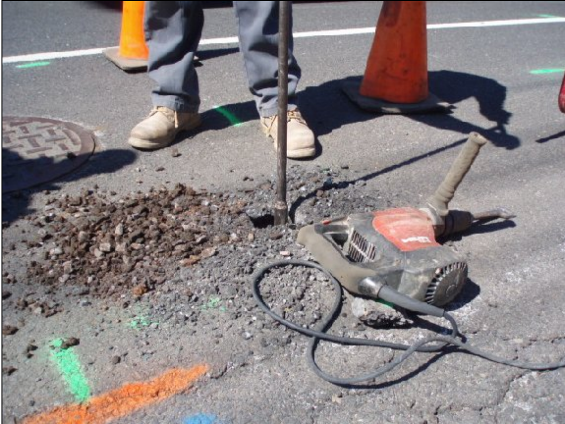
Fig. 2. Starting soil boring next to the manhole at the New Brunswick, NJ, Site.
