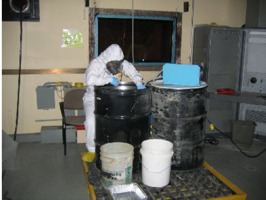
Fig. 3 – Draining leaded-glass windows at the Pluto facility.
