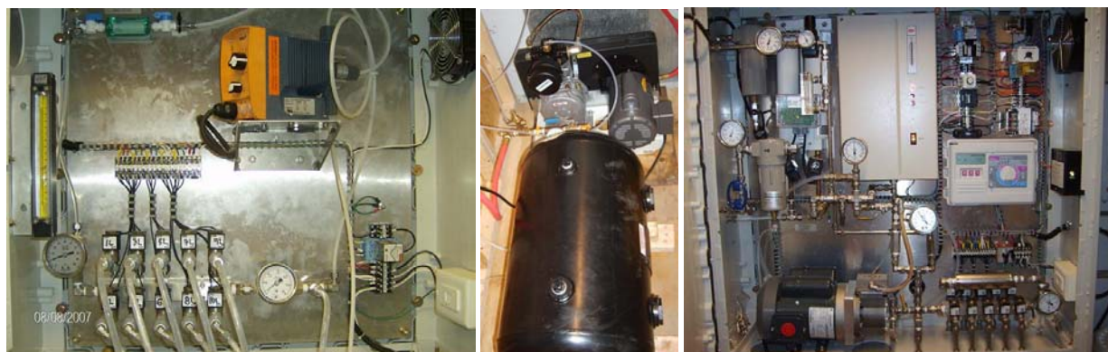
Liquid Peroxide Pump Panel
